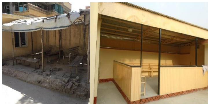
Figure : Kabul Urban Health, Health Facility Waiting Area | before renovation (left), after renovation (right)
